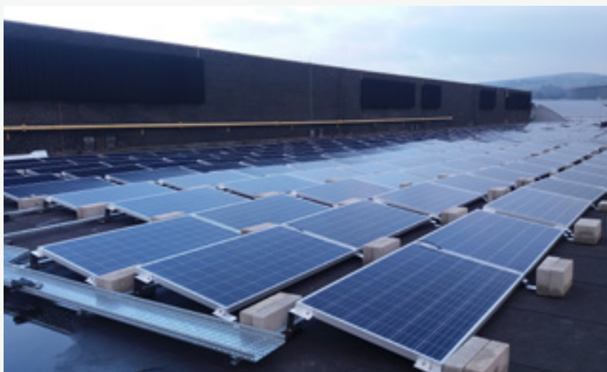
Macclesfield solar panels
